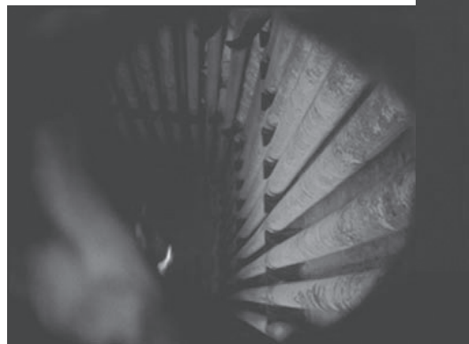
Fired Heater Tubes
