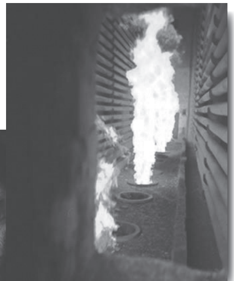
Gas Burner in Fire Box
