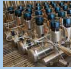
MANIFOLD OF VALVES - DAIRY
